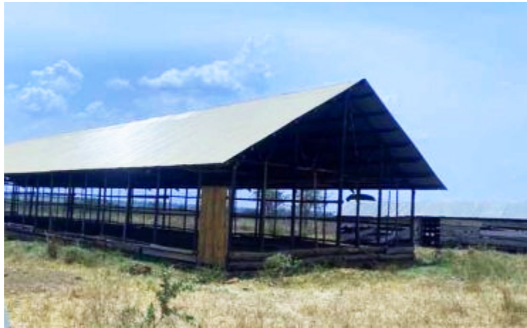
One of the structures constructed using OPM 'Mabati' at a private farm of a senior government official in Kayunga District (Source: New Vision e-paper)
